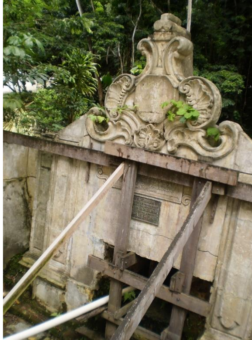
Figure 5 - Degrading situation of the pediment built in the 18th century to identify the Tambiá Fountain, richly carved in limestone with baroque elements.
